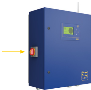
Main switch disconnecter on the iQ-Control Panel
